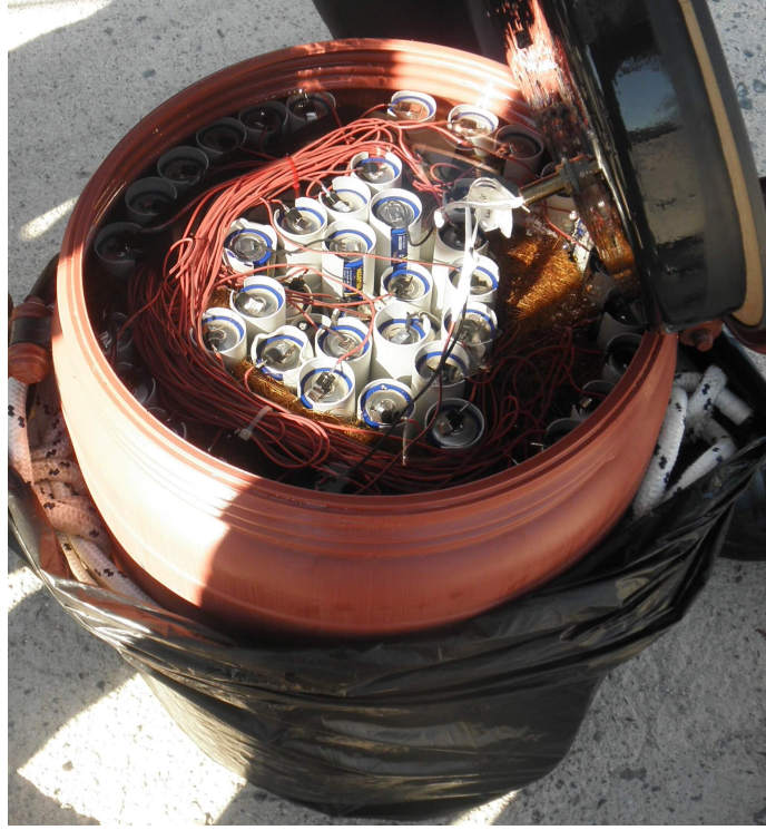
Figure 4.7: A power unit of the GRBNeT Prototype
